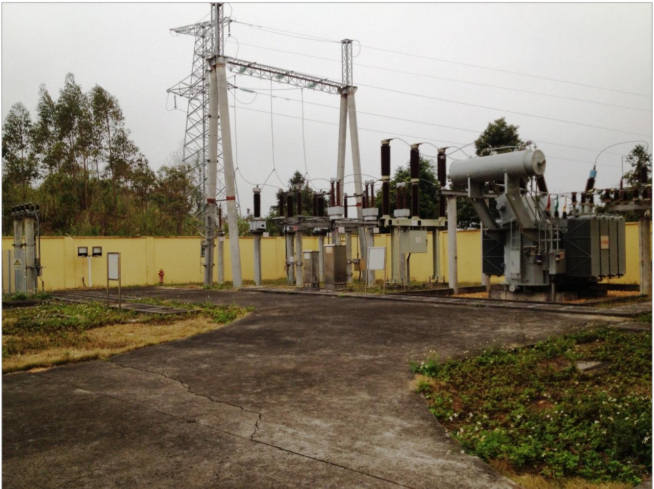
Figure 18.5 GC mine substation
