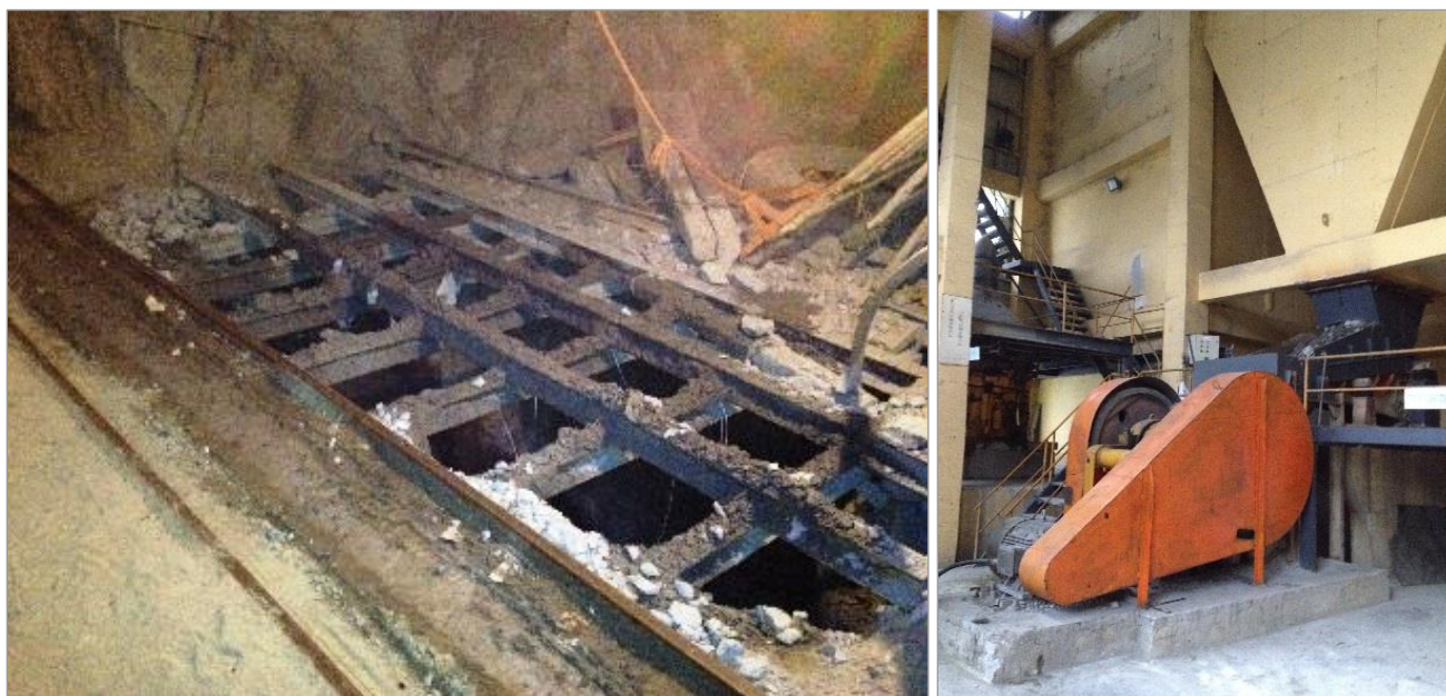
Figure 17.3 Surface grizzly feed to ROM ore bin
