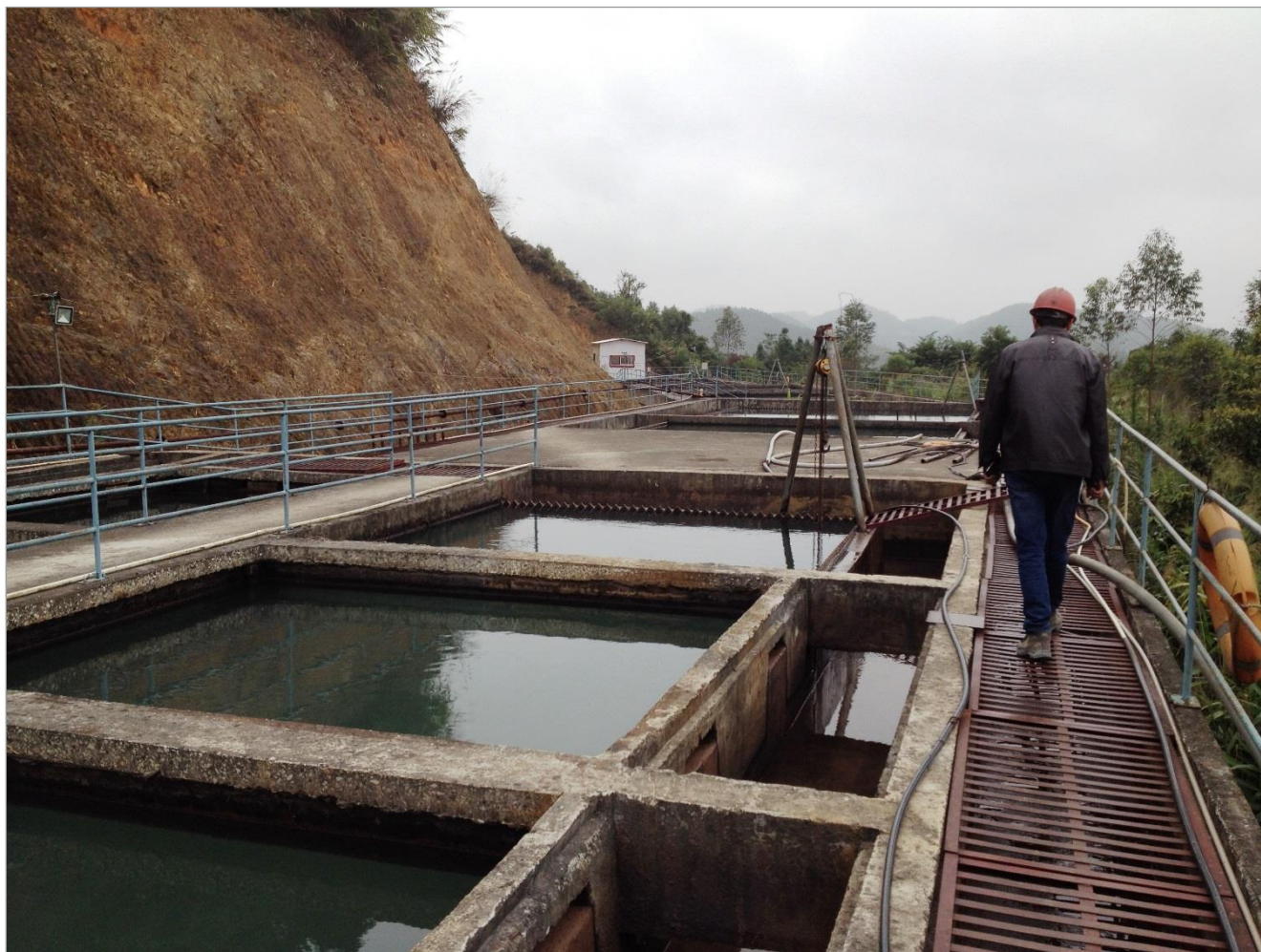
Figure 18.6 GC water treatment facility
