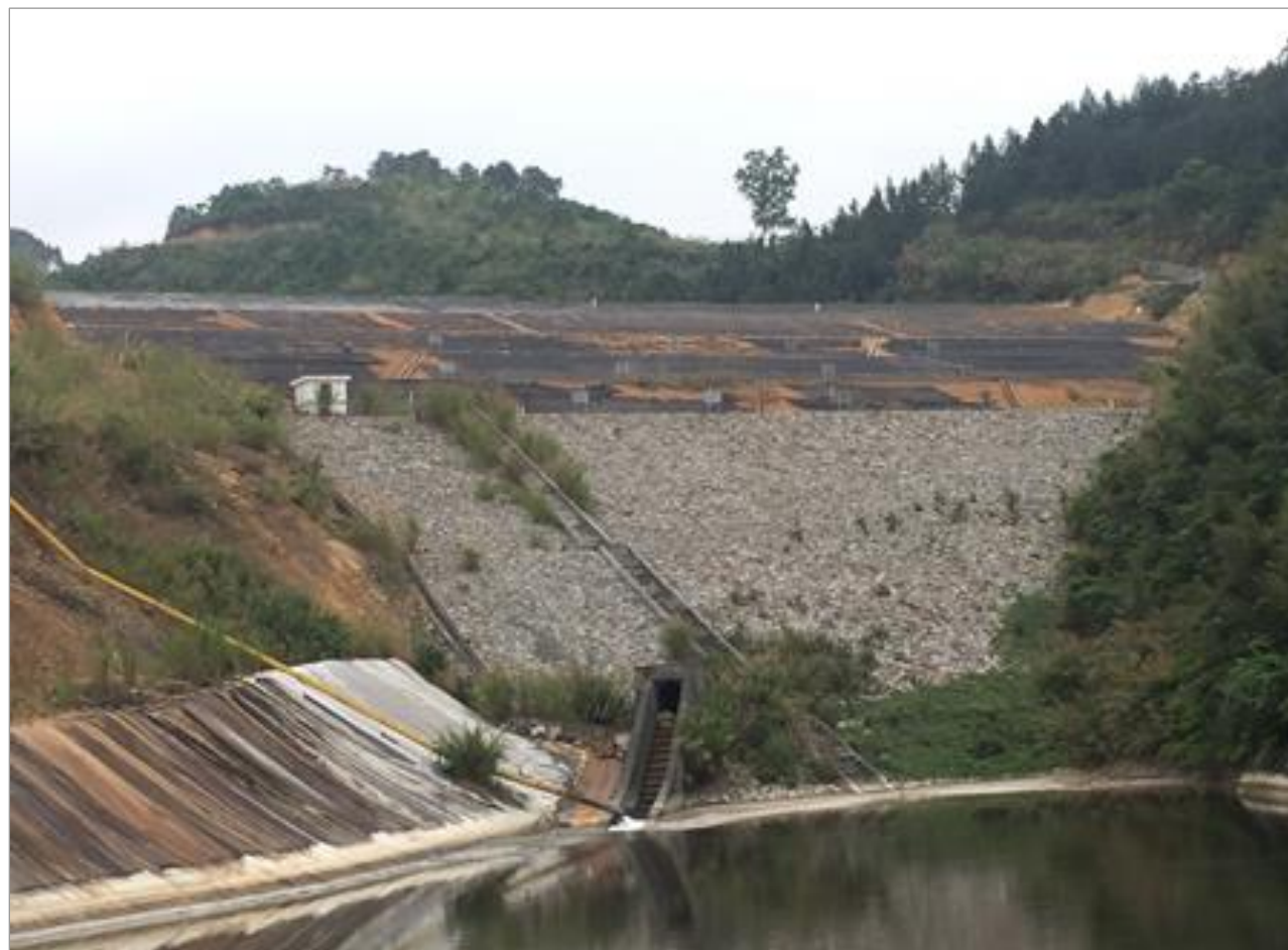
Figure 18.3 GC TMF dam and water seepage
