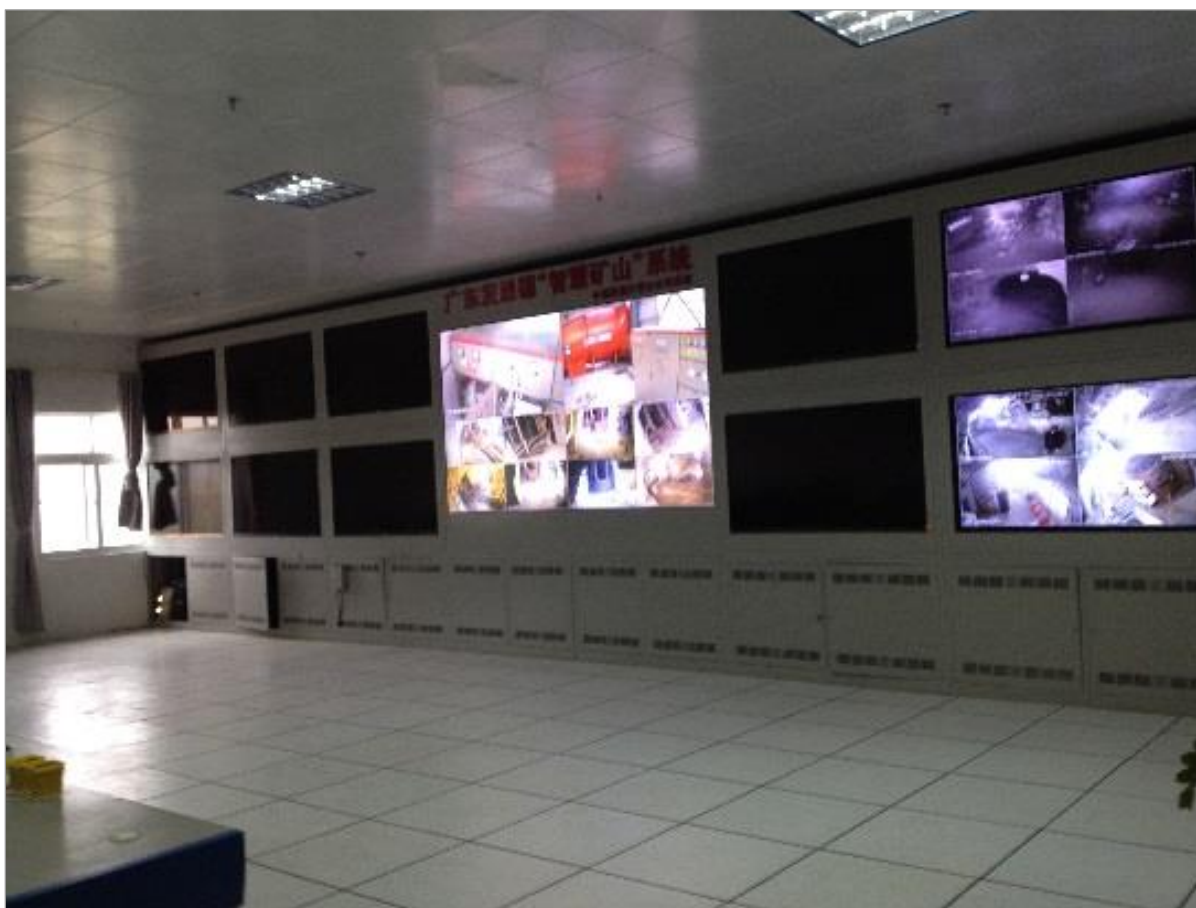
Figure 17.8 Control room screens
