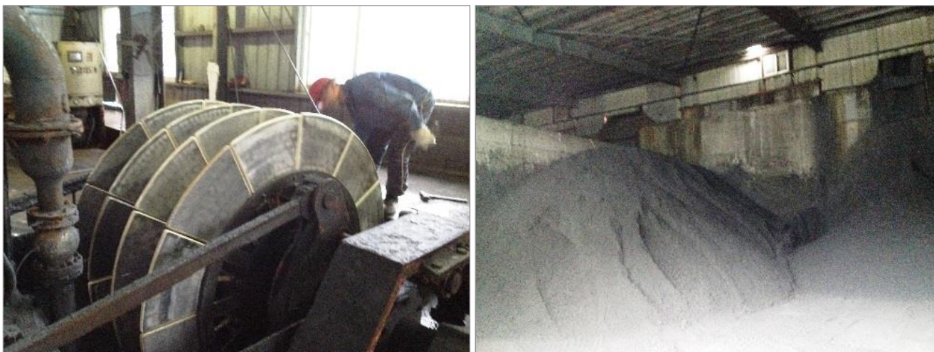
Figure 17.7 Disc filters and zinc concentrate shed
